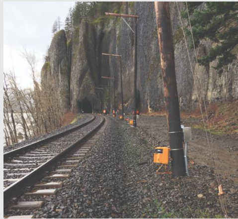
Rockfall Monitoring System
