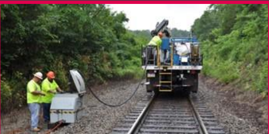
Equipment service and maintenance
