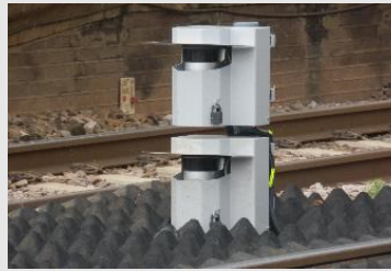
LIDAR used to Detect Debris at Crossings
